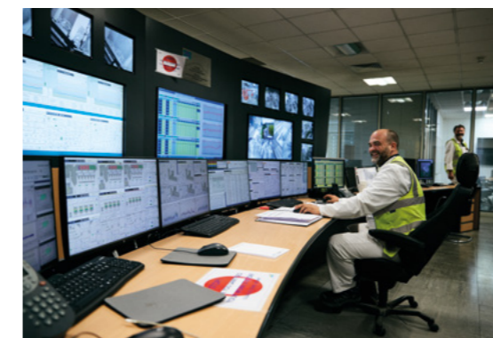
➡ The central control room at Riverside in Belvedere is manned 24 hours a day, 365 days per year.
